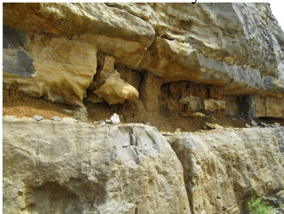
Erosion on Cecil Ashburn Dr.
